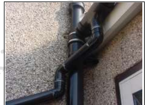
Plastic downpipes with wide joints, we assume that these leak
