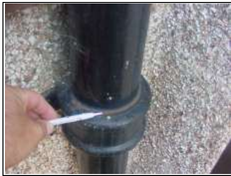
Minor rusting on soil and vent pipe that is expected on cast iron
