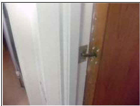
Perko door closers. These indicate loft conversion has been carried out legally
