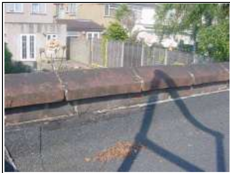
Parapet wall needs re-pointing
