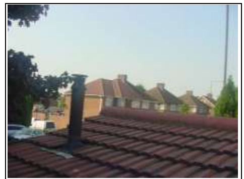
Flue from the boiler in the kitchen
