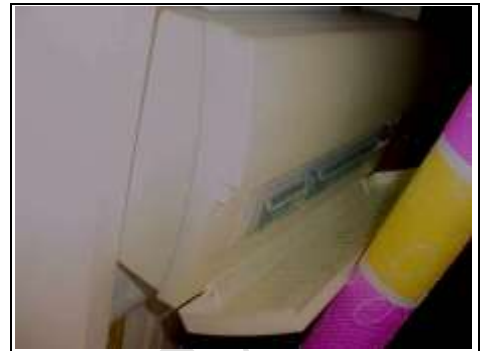
Dated fuse board
