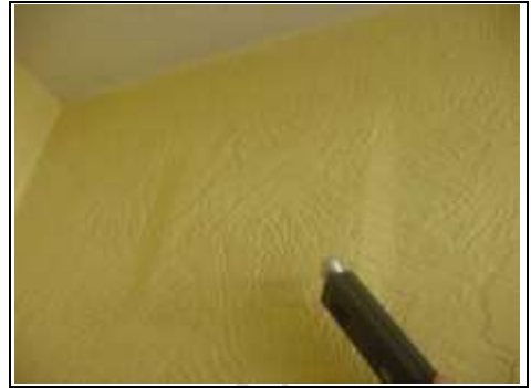
Internal air vent wallpapered over
