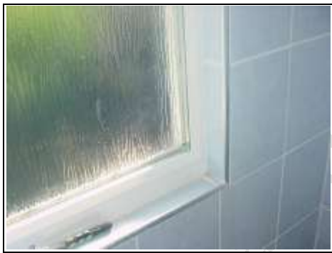
Thin walls in loft conversion (en-suite shower room)
