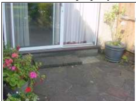
Patio doors with blocked air bricks
