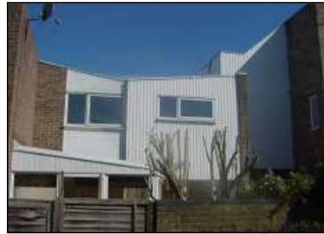
1970's property with cold bridging to the roof beams and the lintels
