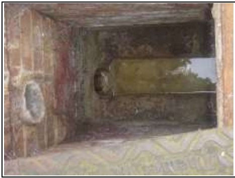
Drain (front) with tree roots coming through (not very clear in photo)
