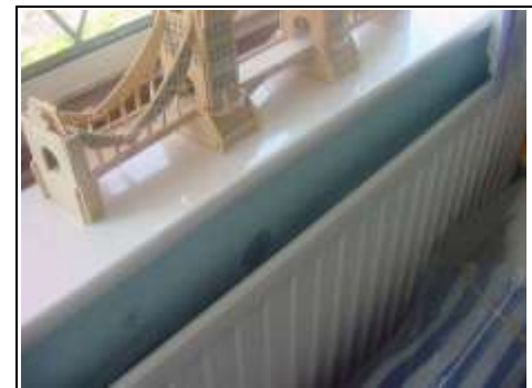
Single panel radiator
