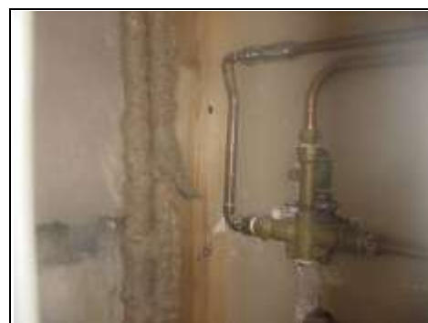
Plumbing visible in cupboard in rear right bedroom. The photo shows valves which can be turned on and off.
