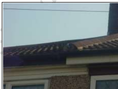
Hog backed tiles between the two roofs that indicate they were put on at different times.
