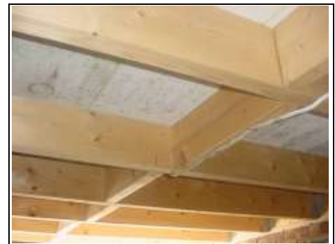
Mould indicates condensation is occurring
