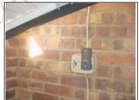
Electrics in the garage
