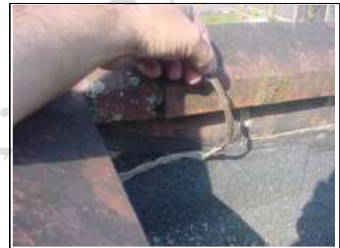
Mastic coming away
