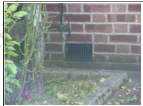
Air brick (front)
