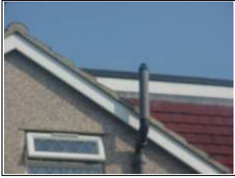
Soil and vent pipe
