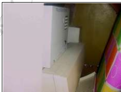
Alarm control panel
