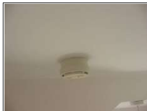
Hard wired smoke alarm
