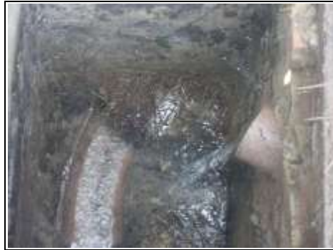
Drain (rear) with tree roots coming through
