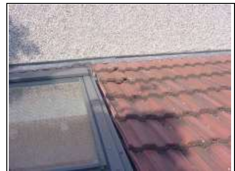
Shallow pitch of roof (remember to keep guttering around roof lights clear)
