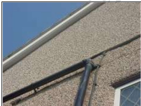
Awkward bend in downpipe
