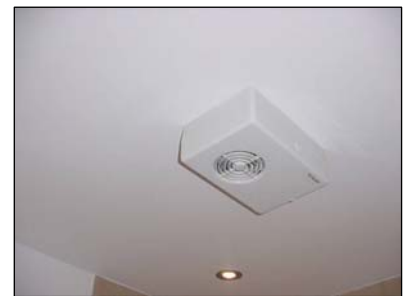
Extract fan Need to identify where the extract fan discharges to
