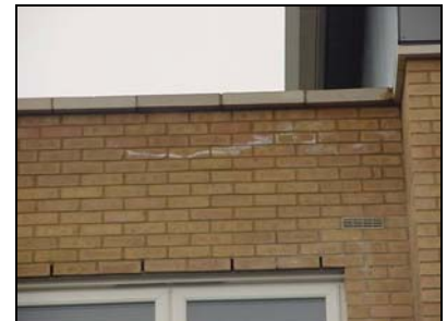
Adjoining properties Efflorescence
