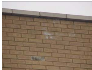
Efflorescence. Also note the weep holes to the lintels above the windows
