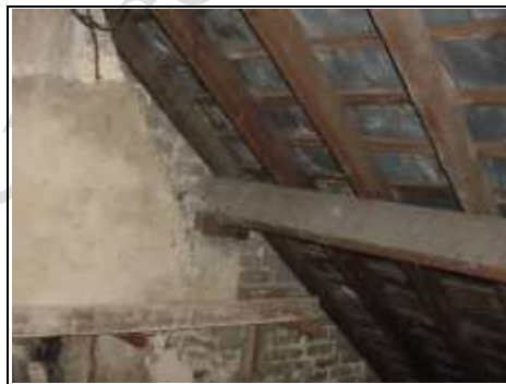
Purlin on rear left hand corner balanced on a brick needs securing
