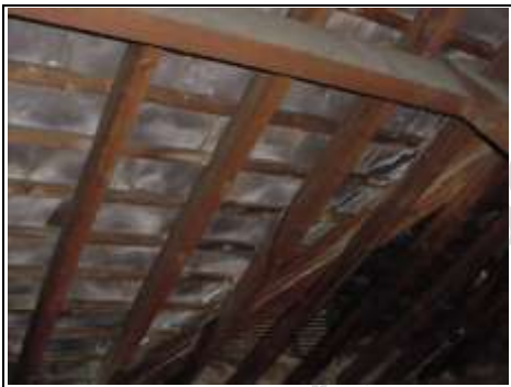
Dampness visible to timbers
