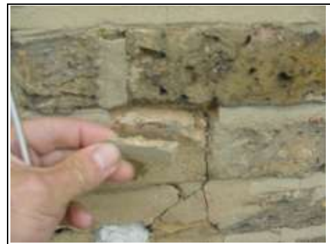
Cement mortar re-pointing breaking away
