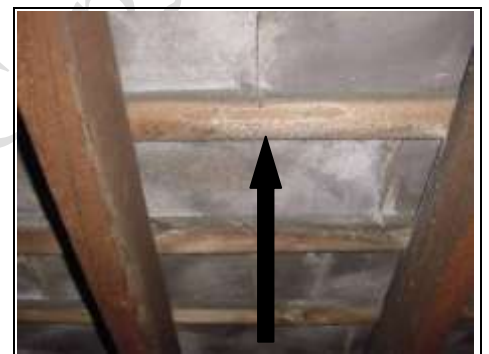
Close up of timber batten showing white salts which is a sign of dampness
