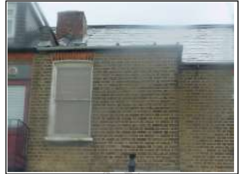
Flat roof we could not view to the rear which looks likely to be a lead roof
