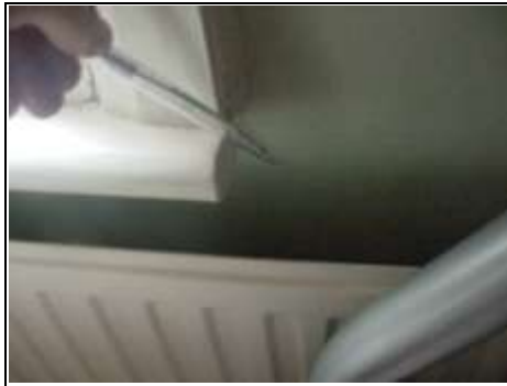
Hairline crack to rear left hand bedroom
