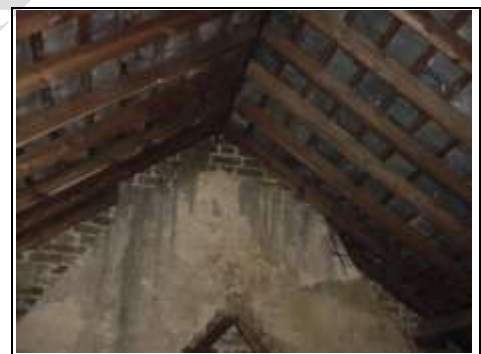
Dampness coming in around chimney to left hand side
