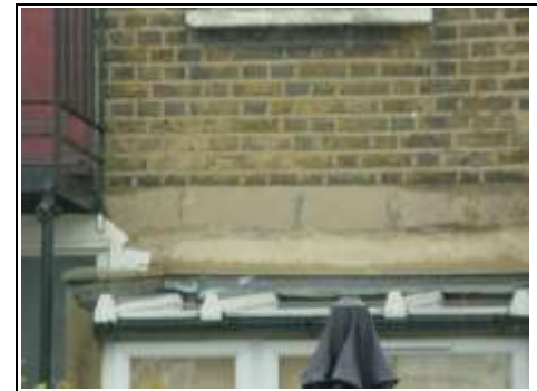
Polycarbonate roof over small conservatory and lead flashing where it meets the building and adjoining roof
