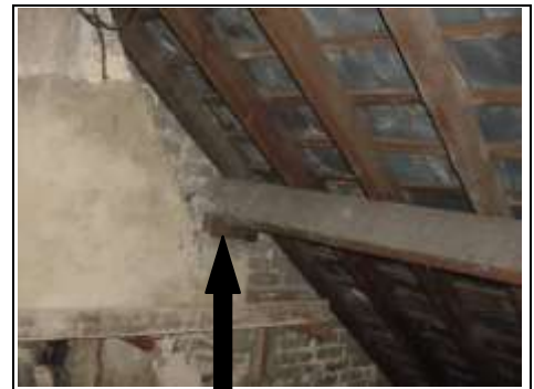
Purlin needs securing at rear left hand corner as balanced on a brick
