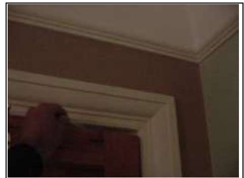
Movement in rear left hand bedroom door
