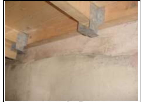
Woodworm or wet rot previously to the floor
