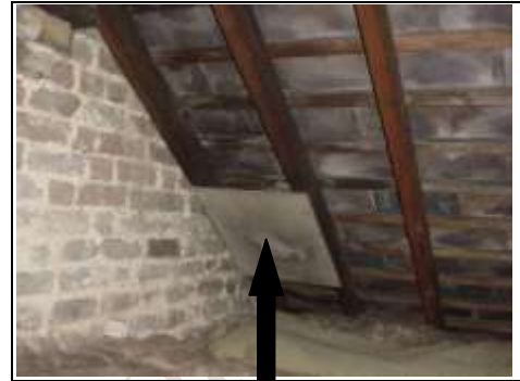
Asbestos to the underside of the roof slates.
