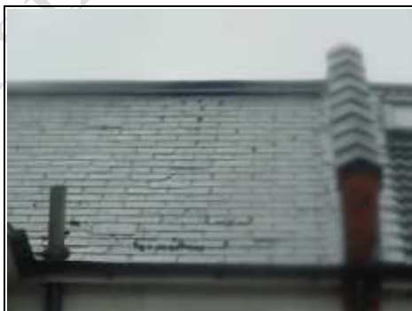
Some displaced and slipped slates to the front of the property
