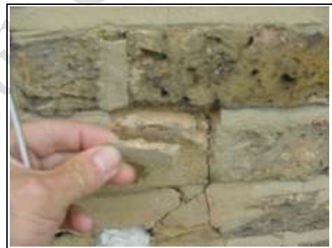
Cement mortar re-pointing crumbling away
