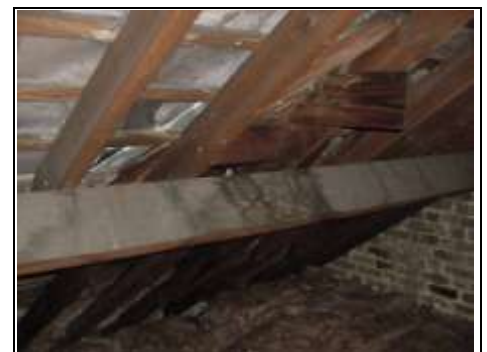
Dampness visible through timbers
