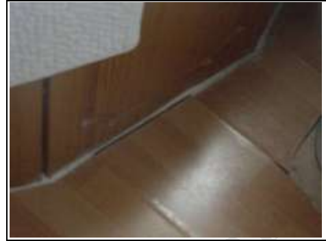
Poor quality DIY laminate floor boarding
