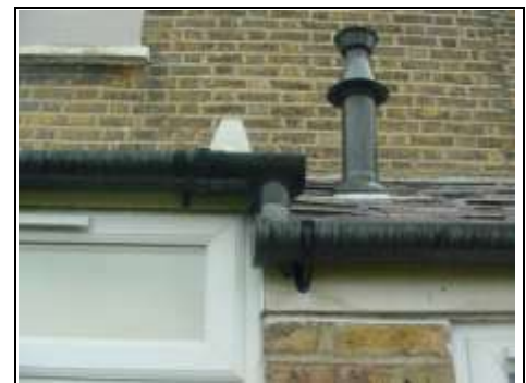
Soil and vent pipe from ground floor cloakroom/WC
