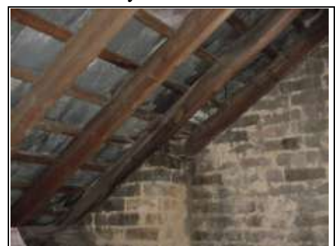
Dampness coming in around rear right hand chimney
