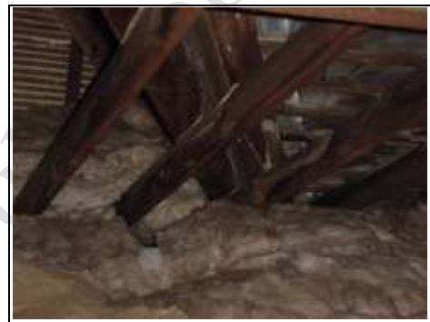
Dampness getting in beneath valley gutter
