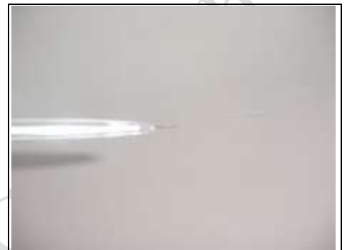
Cracking in plaster front left hand bedroom
