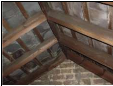
Dampness visible to underside of some of the slates
