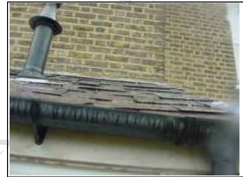
Poor quality slate to rear low level roof
