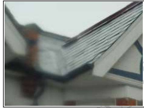
Photo of roof with raindrop on it showing perimeter has lifted slightly
