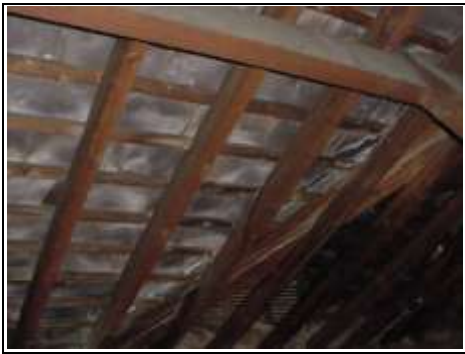
Dampness visible on timbers
