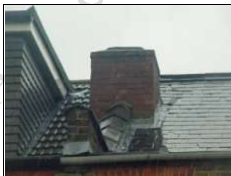
Rear right hand chimney (lead looks to be cut straight rather than following the brick joint)
