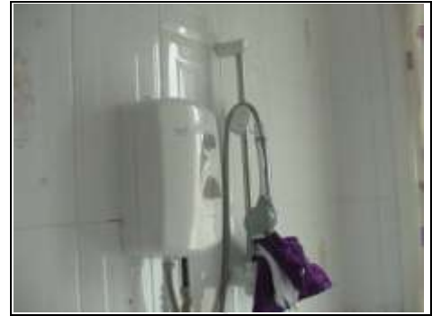
Shower water heater
