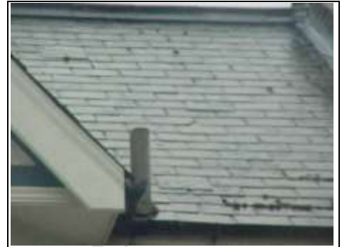
Possible asbestos flue to front right hand side
