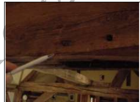
Two peg joints on beam where brace is missing
