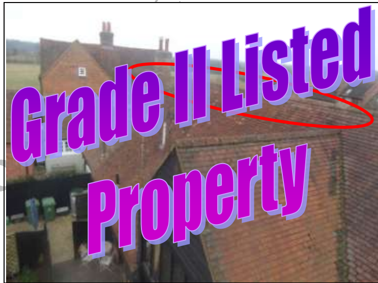
Gaps in ridge tiles
