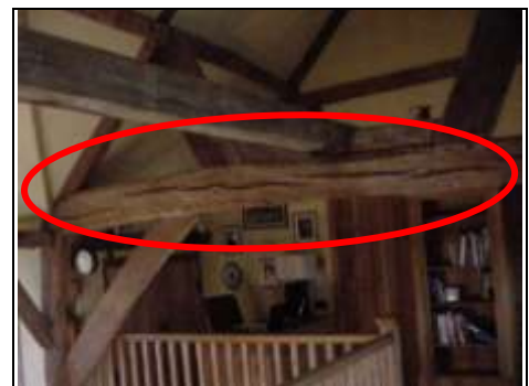
Gallery style landing, cracks in roof timbers
