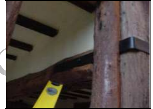
Bare timber visible in some areas
