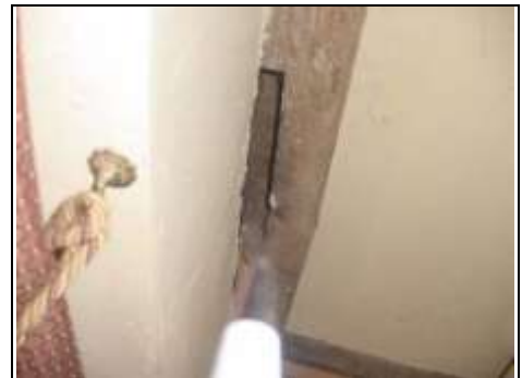
Top of stairs where the brace is missing
