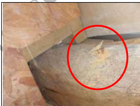
Signs of woodworm to purlin on right side of roof
