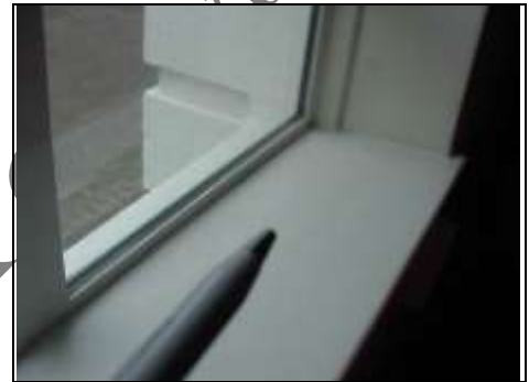
Condensation/water staining on the window sill
