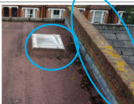
Left parapet wall and roof window leaking
