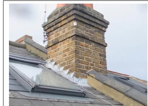
Problems to base of chimney
