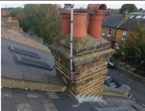
Water trap behind chimney
