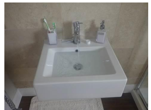
Sink in top floor shower room slow to drain
