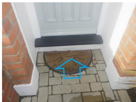
Front air vent acting as gutter
