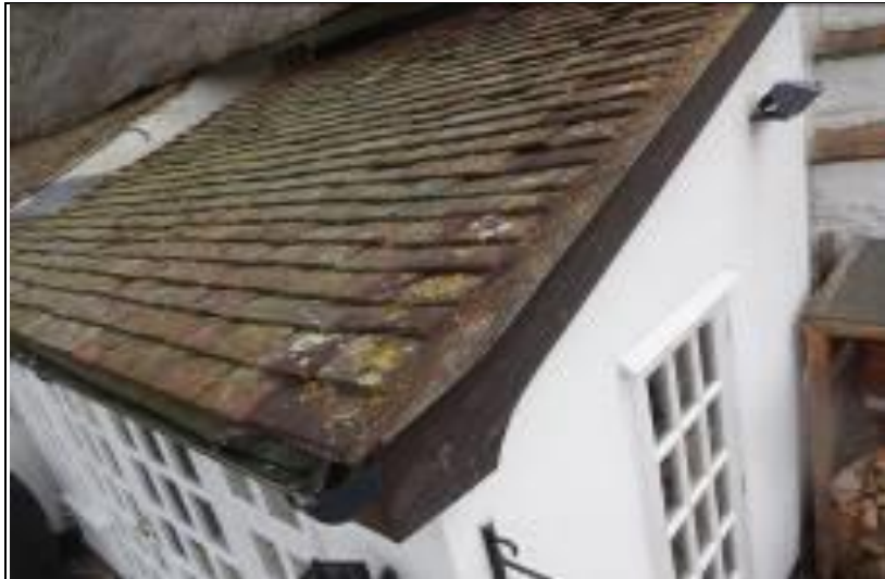
Spalling to tiles ~ Aerial View - 360 Photo ~
