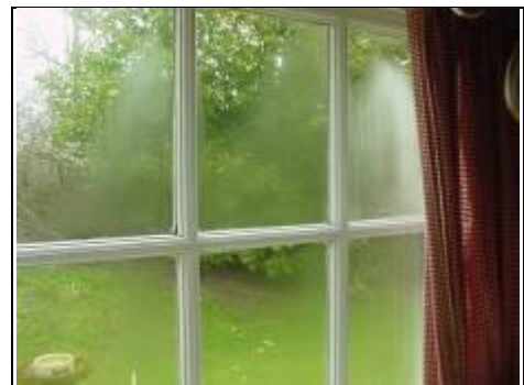
Condensation to windows in kitchen
