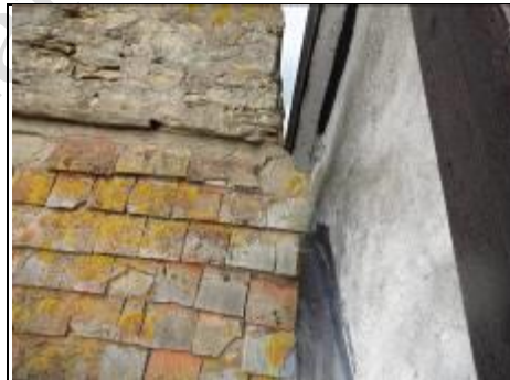
Gap between chimney and main building
