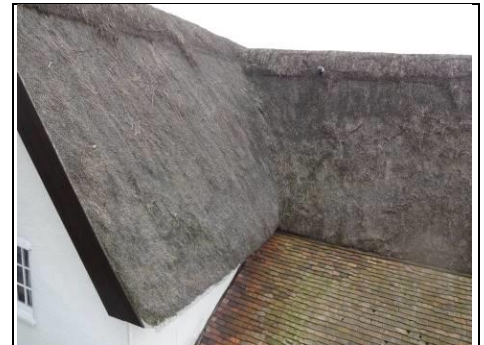
Thatch in poor condition
