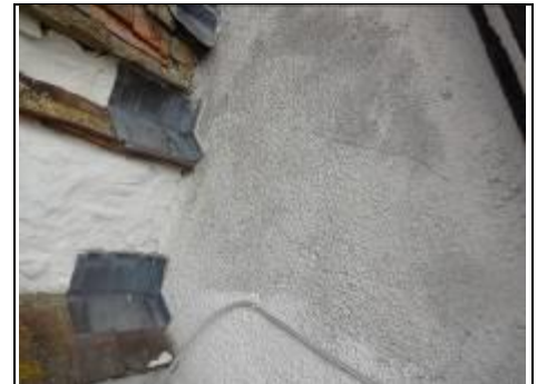
Mastic on lead to right gable
