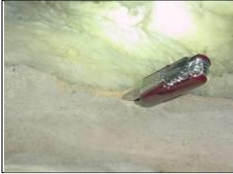
Woodworm/rot in timer in middle roof where it meets left roof
