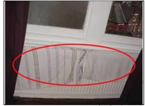
Drying washing on radiators can cause condensation
