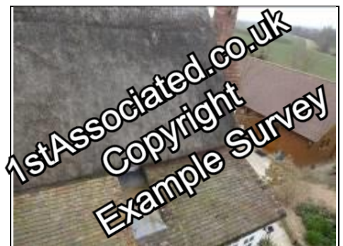
Displaced tiles and in need of repair
