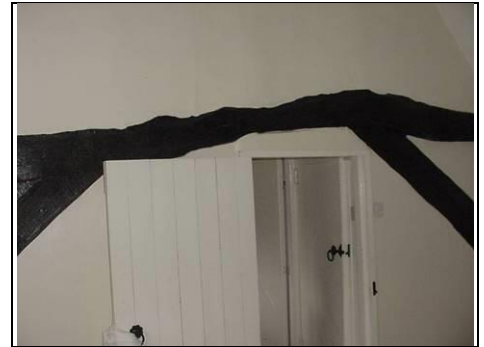
Ledge and brace door and timber clad door
