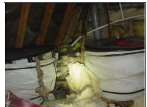
Water tanks in middle roof
