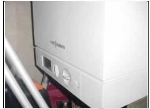
Viemann Boiler in services room
