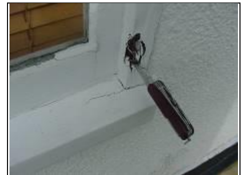
Knife test in rotten window
