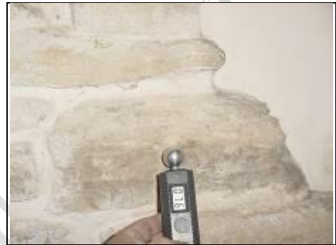
Dampness in stone
