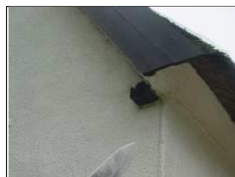
Purlins can be seen protruding out of walls which can lead to rotting
