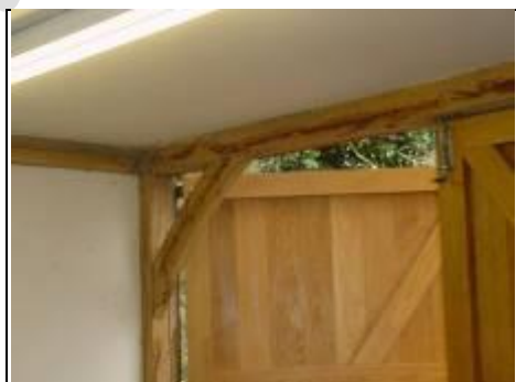
Dampness coming into garage
