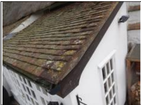
Spalling to tiles
