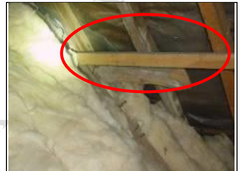
Purlin missing replaced with very thin purlin Plastic sheeting
