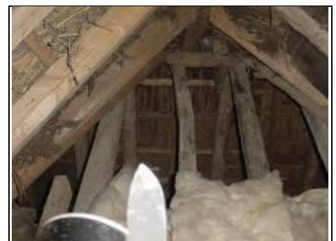
Deterioration/twisting to timbers in left roof
