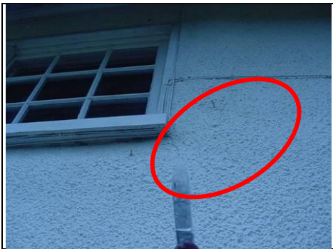
Cracking to the window
