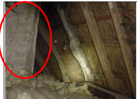
Hidden chimney/smoke hood
