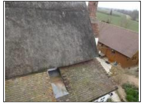
Displaced tiles and in need of repair
