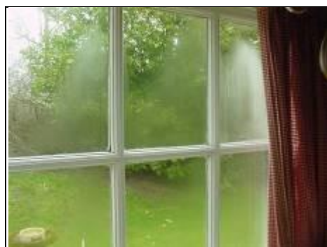
Condensation to windows in kitchen
