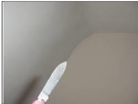
Hairline cracking in master bedroom
