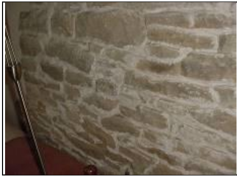
Dampness coming through and various repairs
