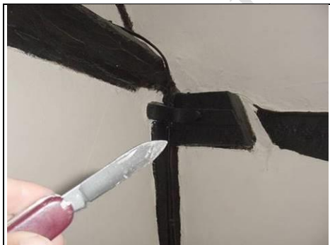
Infill panel with metal brace
