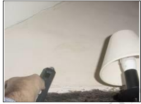
Dampness coming through plaster in right bedroom
