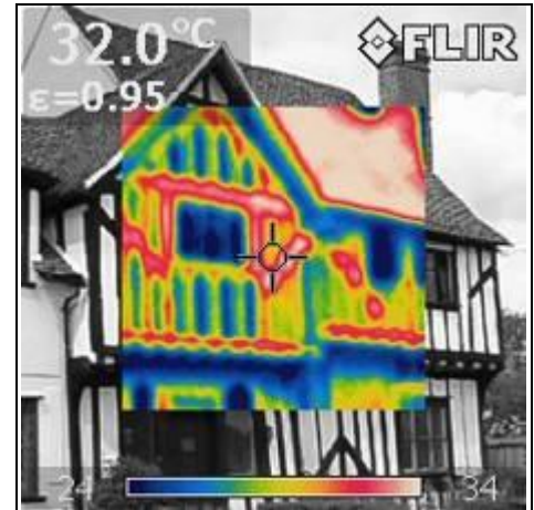
Timber framed Public House Thermal image showing heat loss
