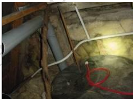
Soil and vent pipe
