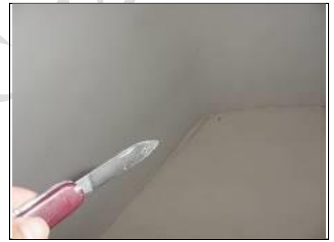
Cracking in far right bedroom
