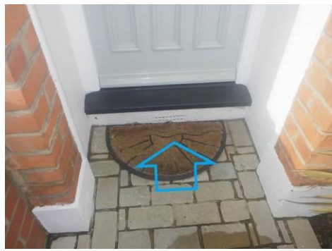
Front air vent acting as gutter
