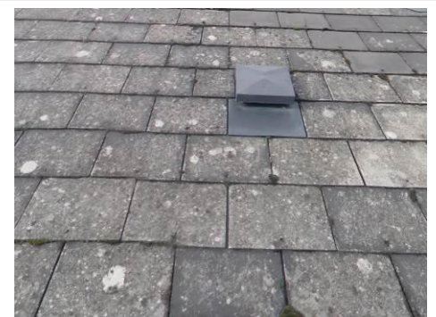
Slates may have asbestos content
