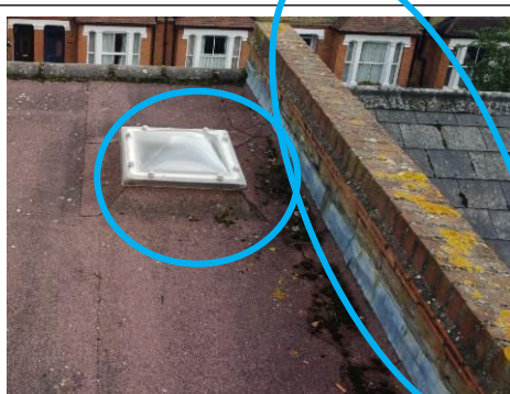
Left parapet wall and roof window leaking
