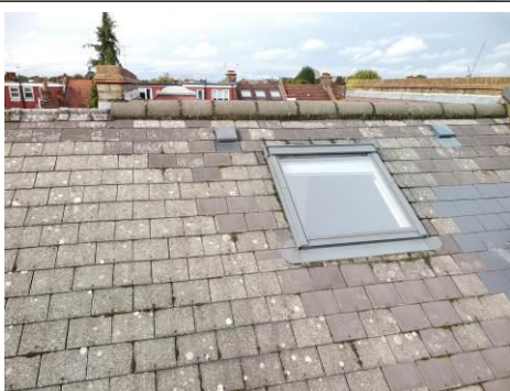
Asbestos roof slates ?
